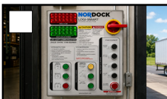
INTEGRATED CONTROL PANEL
