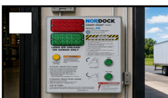
RESTRAINT CONTROL PANEL
